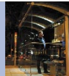
Bus Shelter Lighting
